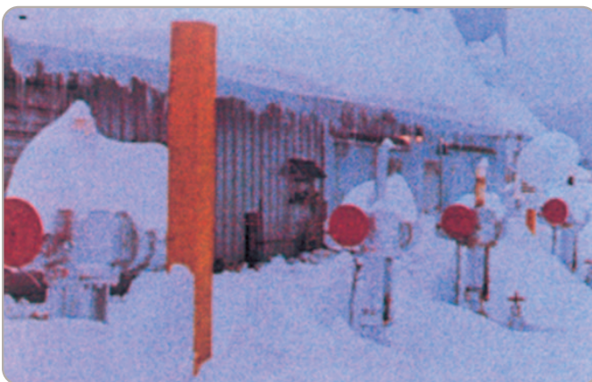
EIM actuators on the Trans-Mountain Pipeline, Canada, withstand temperatures of -40° F (-4° C)!
