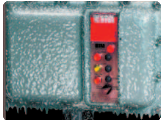
Lab workers at McKinley Climatic Lab, Eglin Air Force Base, needed reliable actuators to operate dampers at temperatures as low as -100°F (-38°C). The only actuator that could do this was the rugged EIM Series 2000.
