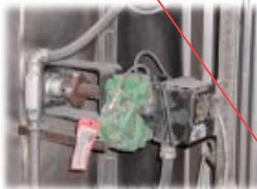
Fuel Air & Aux Air Drives
